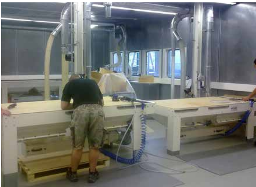
Two Expert Z 20 sanding dust extraction tables in the paint preparation
