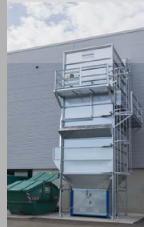
Storage of paper dust simple and safe. The BrikStar C in a print shop combined with a MultiStar filter.
