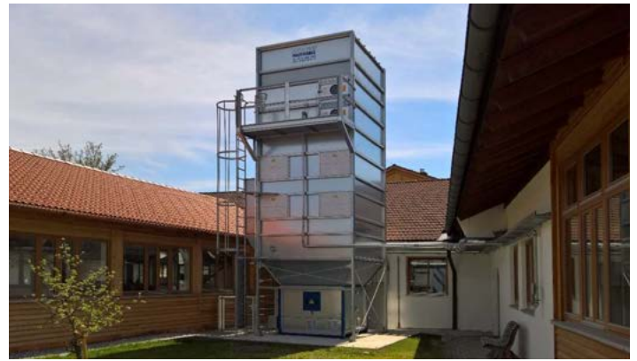
MultiStar filter system with BrikStar briquetting press as the discharge unit
