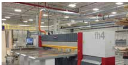
Machines coupled via automatic gate valves
