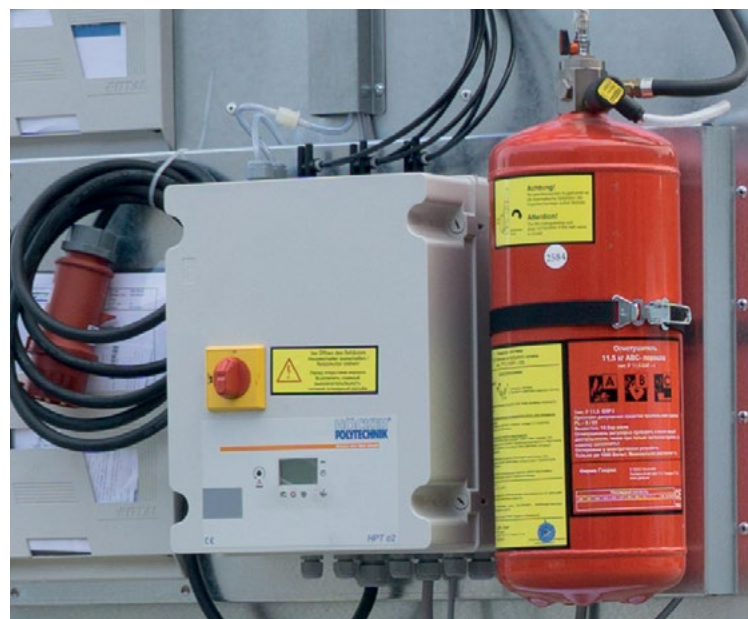
Fig. below: PLC-control, automatic fire suppression system
