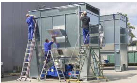
Assemble extinguishing pipe, flame deflector, cleaning control and connect motors. All done.
